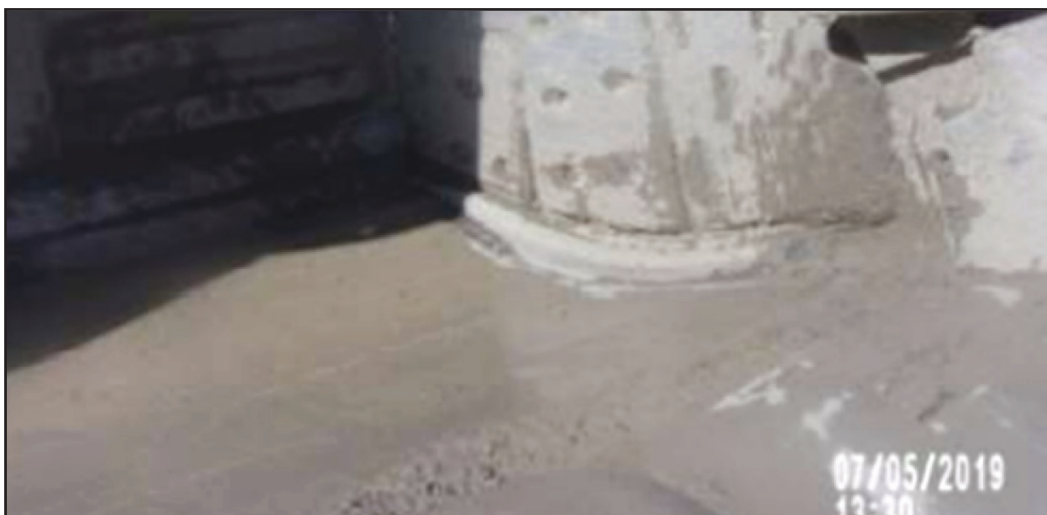
FIGURE 8: CCO wear package field service evaluation inside floor (JCB-Gearvest (Pty) Ltd, 2019)
